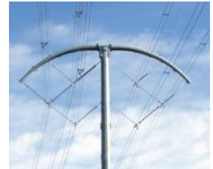
BOLD Transmission Line
