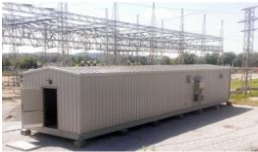
Drop in Control Module
