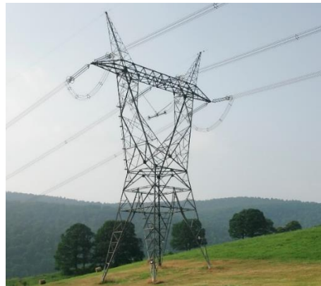
765 kV Transmission Line
