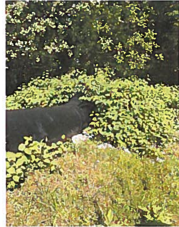
Photo 10- Atypical view of the overflow pipe showing encroachment of vegetative growth at the outlet of the pipe. This area is scheduled to be cut and the vegetation is to be removed.
