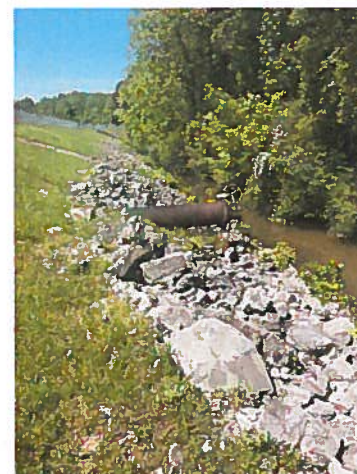
Photo 6 – Typical view of a former discharge pipe. No seepage was observed around the pipe.
