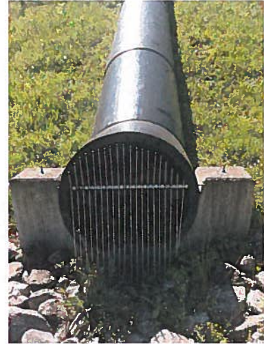
Photo 8– Typical view of 36 inch diameter overflow pipe showing good conditions with no obstructions to flow and no visible erosion along the pipe.
