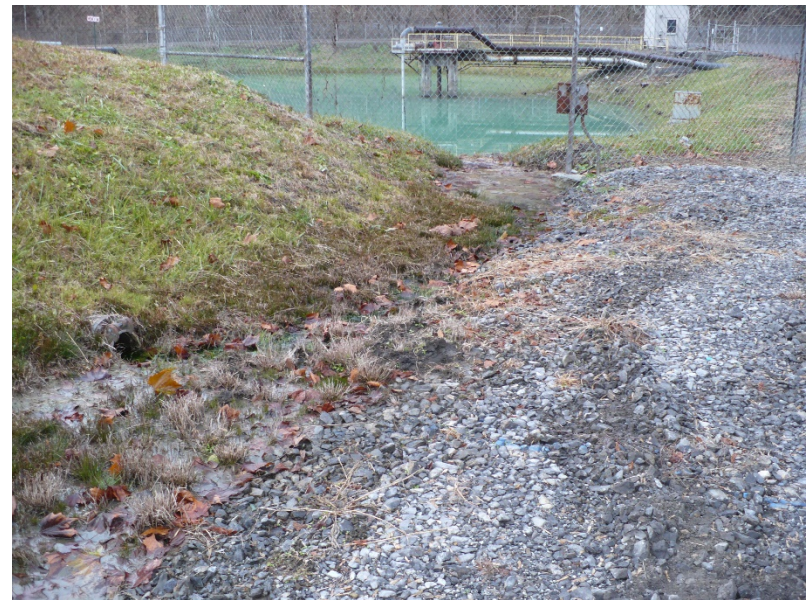
Photo #8 – seepage leading towards weir #5
