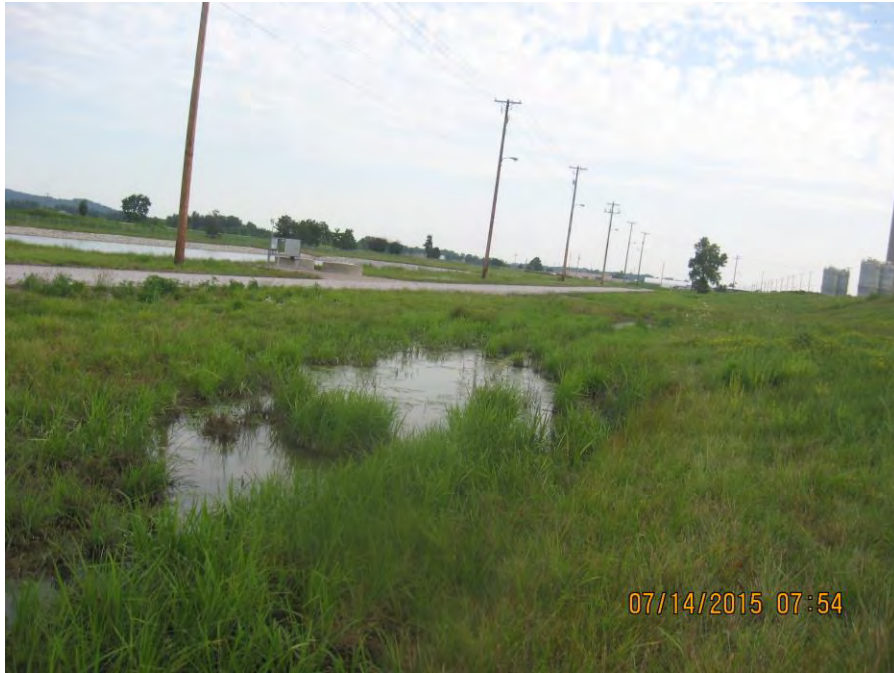
Photo 3: West Bottom Ash Pond, west dike: ponded water at exterior toe.
