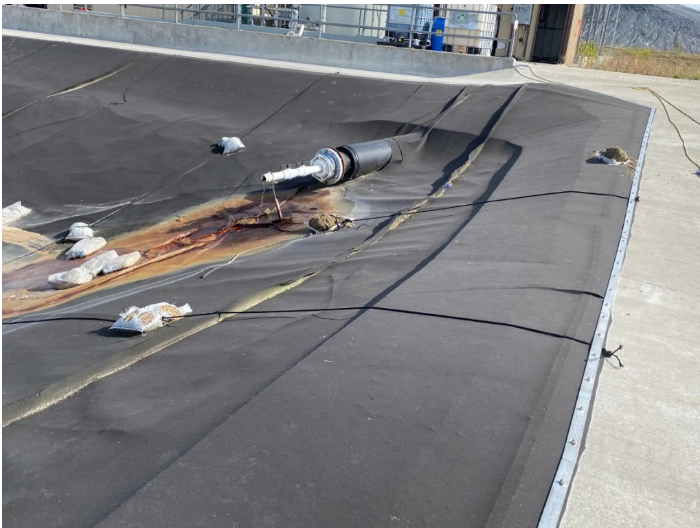
8. Leachate inlet pipe at the southeast corner of the leachate collection pond.
