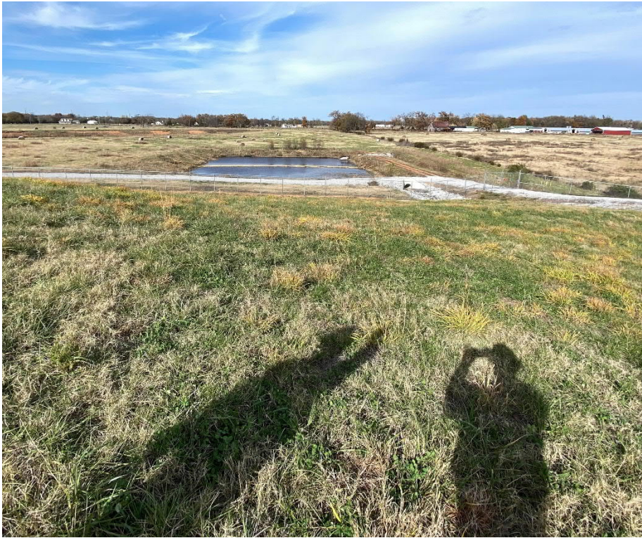
15. Fabriform letdown at the northeast corner of the landfill that flows into the north sediment basin.
