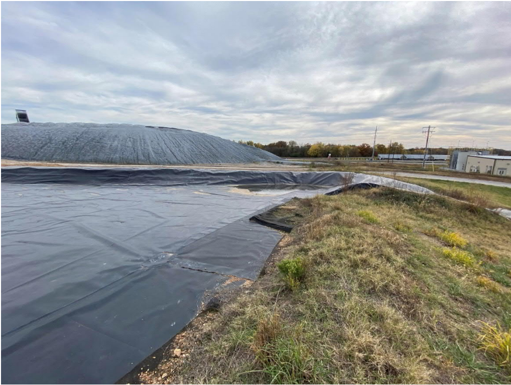
5. Minor ponding at the top of the southwest letdown of the inactive area.
