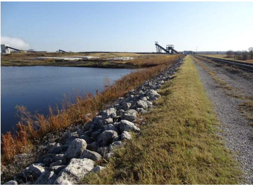
Photo #9 - Vegetation growing in the riprap on the south embankment
