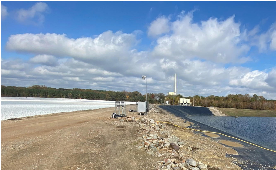
5. Underdrain pumping controls on the west side of the leachate collection pond.
