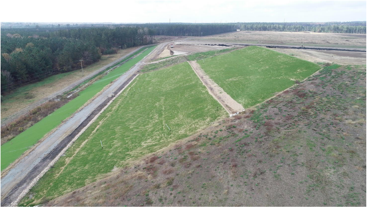
10. The closure turf test pad located on the south side of Cell 1.
