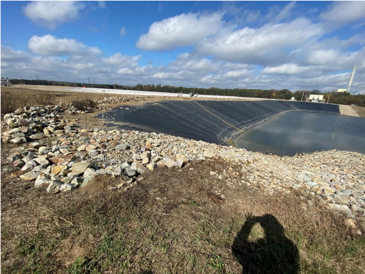
4. The west side of the leachate collection pond that has the geomembrane rub sheet.
