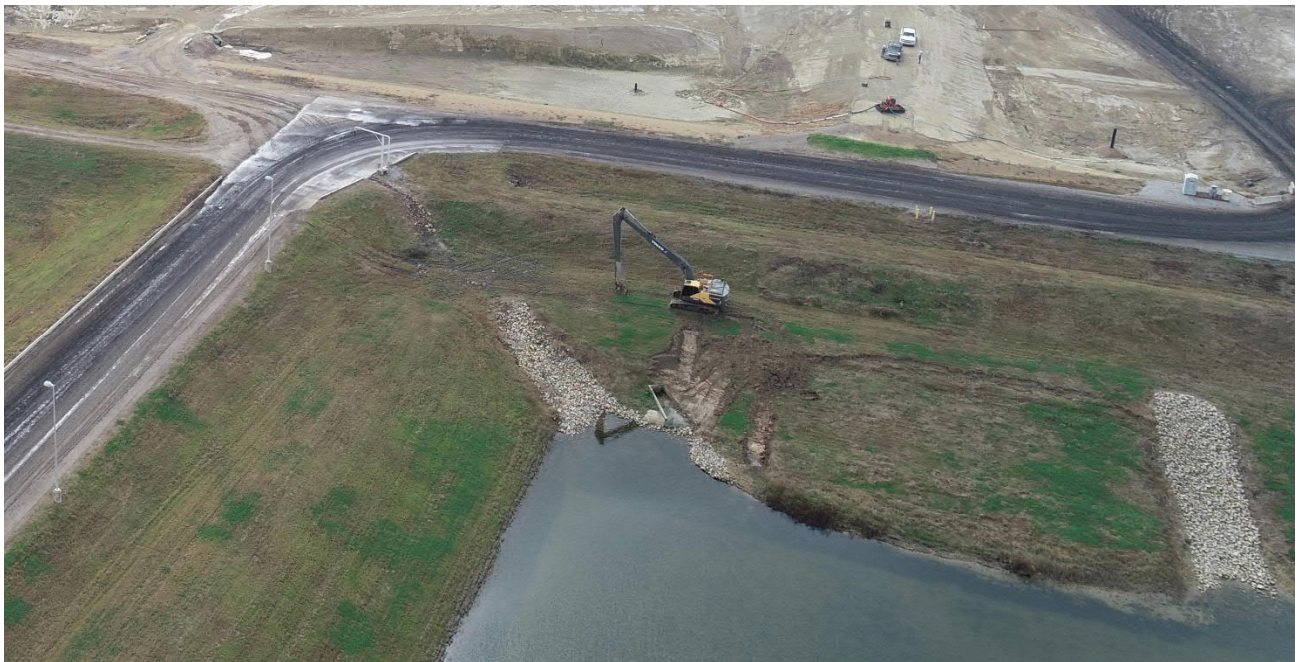
2. The southeast corner of the leachate collection pond that is being repaired.
