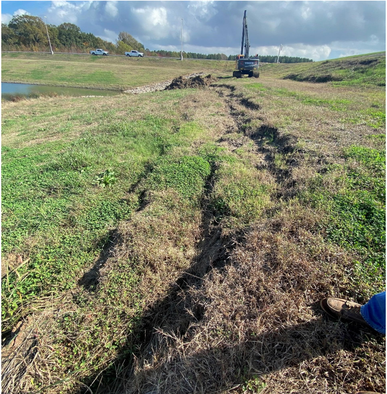
3. Sloughing on the southeast corner of the leachate collection pond looking towards the east.
