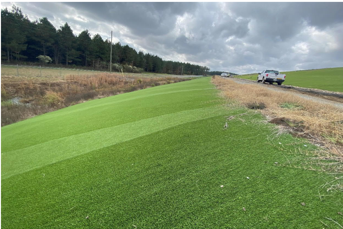
9. South side berm that is covered with artificial turf below the closure turf test pad.
