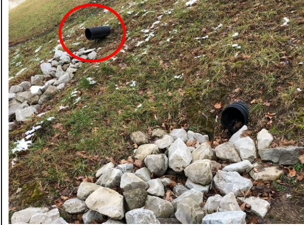
Photograph 10: View of the leachate detection outlet and underdrain outlet for the north area leachate holding basin.
