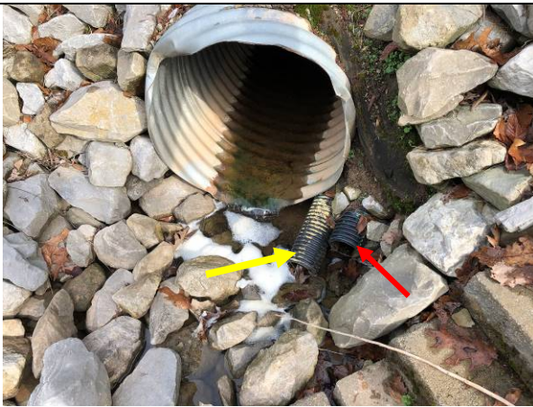
Photograph 11: View of the primary spillway outlet for the south valley sediment collection pond and the leachate detection & underdrain for the south valley leachate holding pond.
