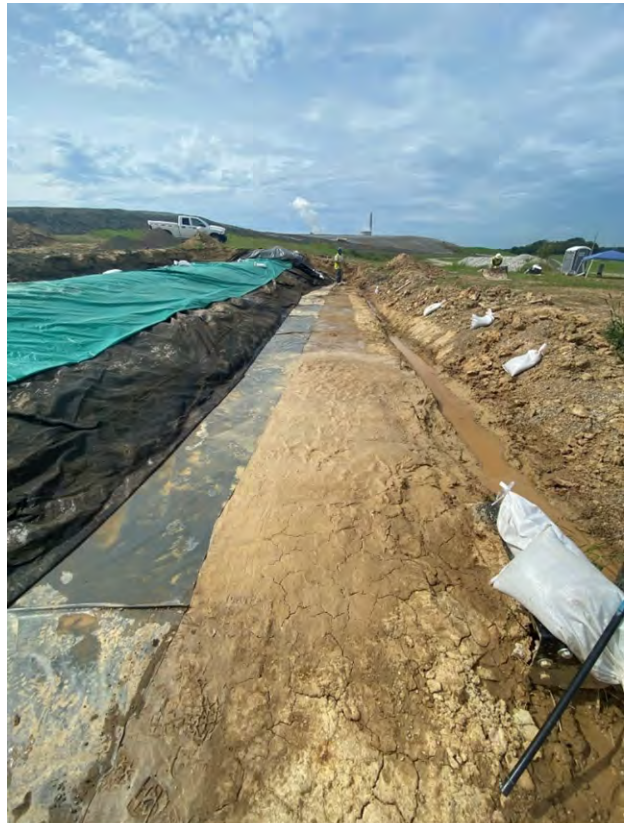
Photo 2: Floor liner and exposed subgrade after rain flap removal.
