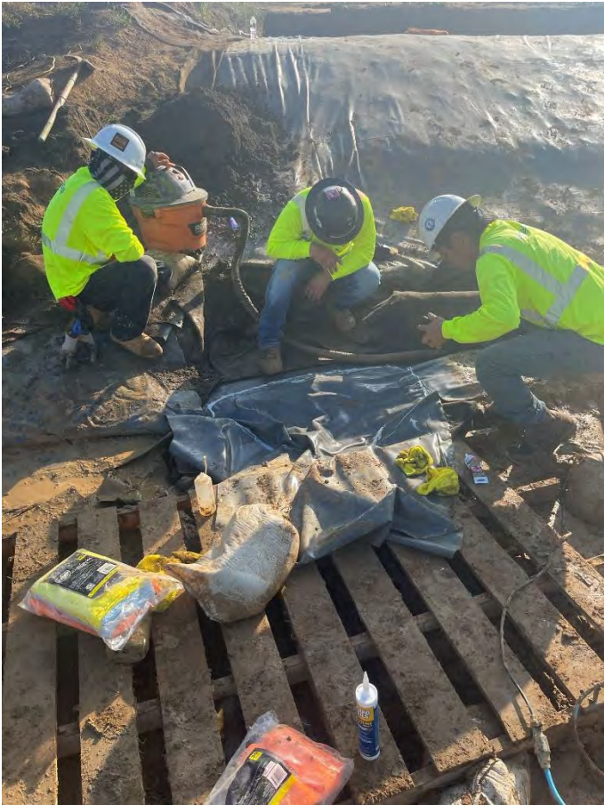
Photo 1: At the north end of the berm CCS is repairing the weld between the existing and new PVC liner.
