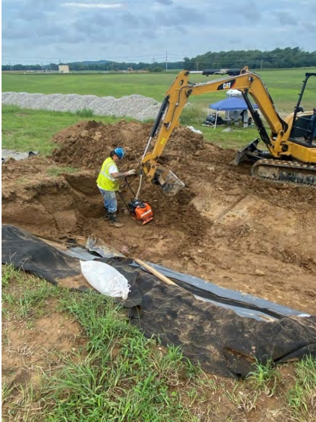
Photo 1: Re-compacting the south end of repair area to create a smoother subgrade after drying the surface in this area.
