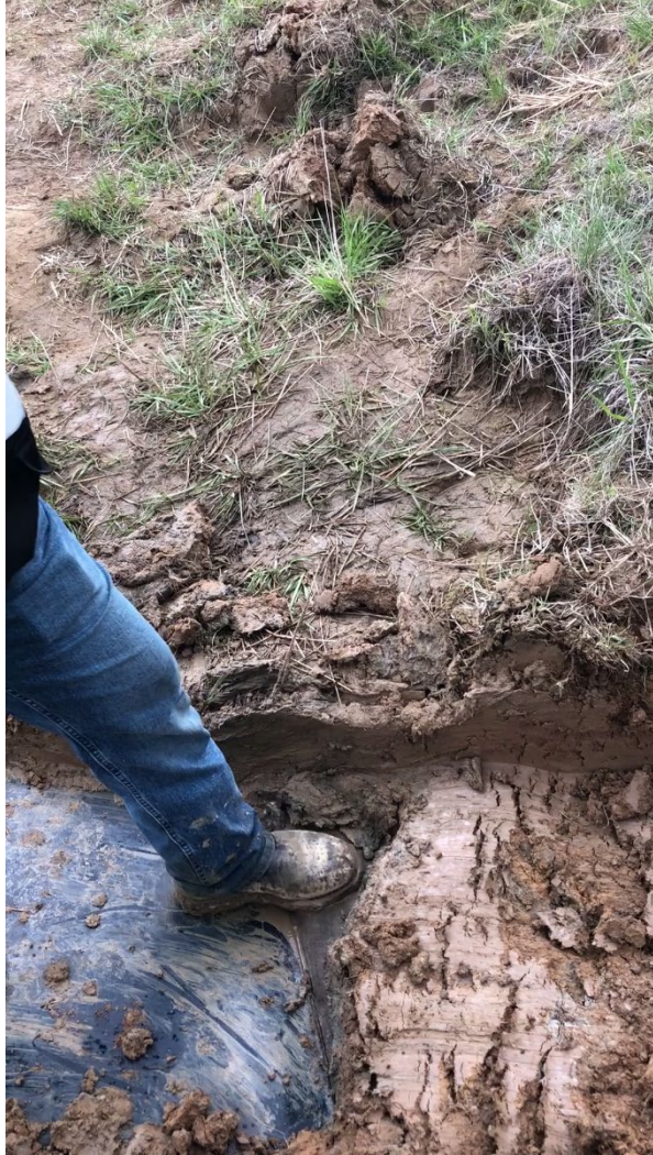
Photograph 6: View of the trapped leachate water between the PVC geomembrane layers of the intermediate berm.
