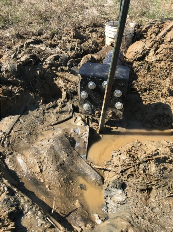
Photograph 1: View of the leachate seepage shortly after initial discovery in the area around Quick Connect #12.
