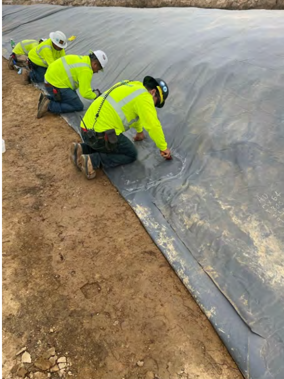
Photo 1: CCS removed and replaced the temporary leister repair at the toe of the berm with an adhesive patch.
