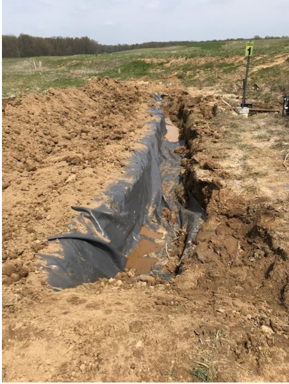
Photograph 3: View of the temporary leachate collection trench excavated upon initial discovery of the leachate seepage issue.
