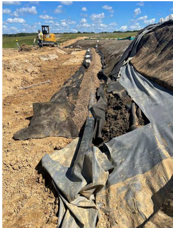
Photo 2: The underdrain pipe was surrounded with stone and wrapped with geotextile. Enerfab used a leister gun to thermal weld the geotextile together at the overlap.
