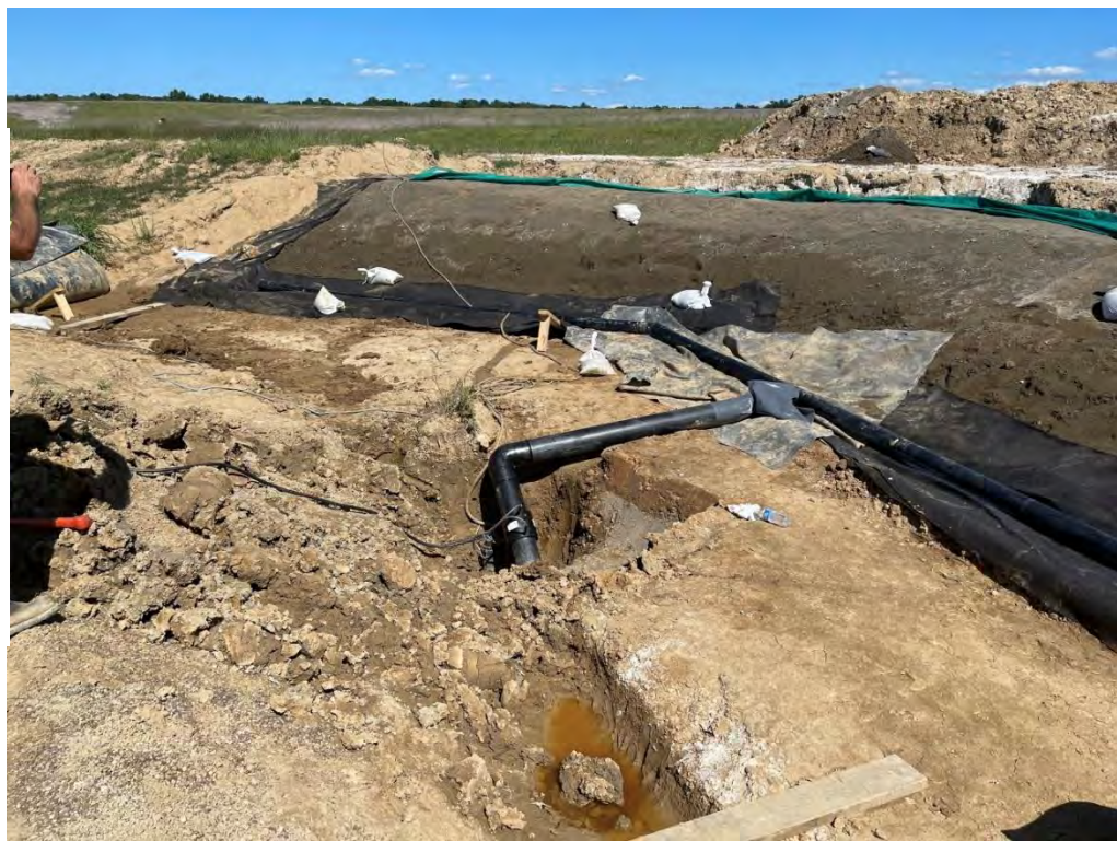
Photo 4: The underdrain has been connected to the leachate trunk line pipe. This photo shows the exposed underdrain pipe awaiting fabric and stone.
