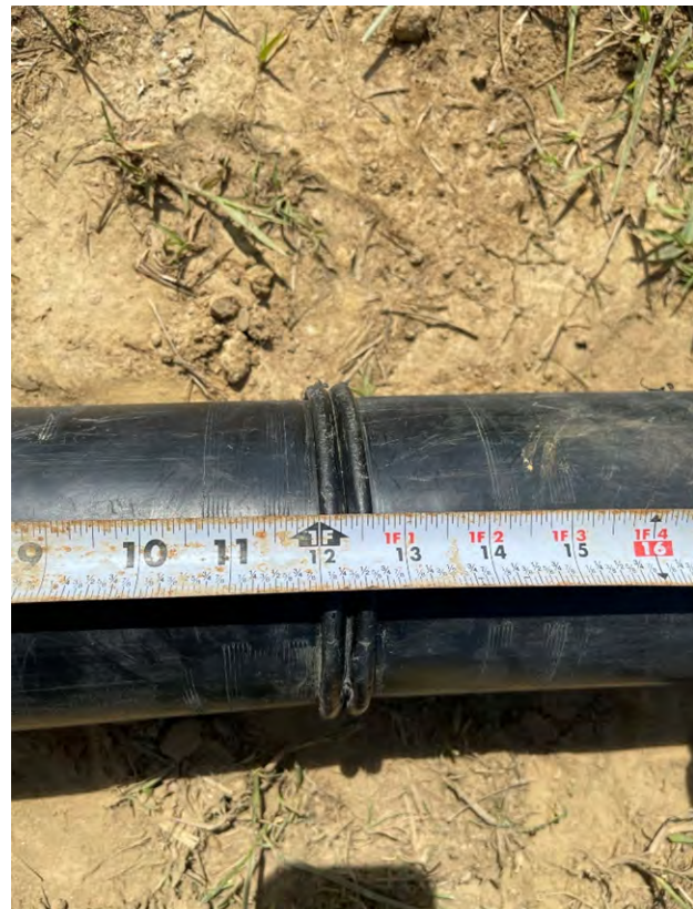
Photo 2: 4-inch HDPE perforated underdrain pipe weld performed off-site meeting minimum bead width of 3/16-inch.
