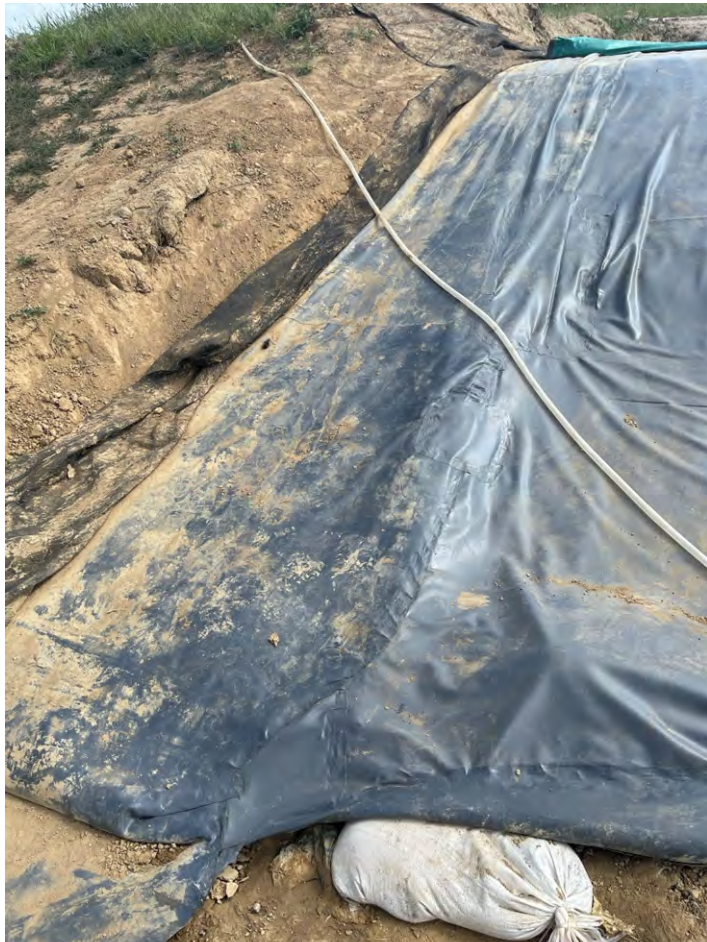
Photo 1: Looking at the north end the existing and new PVC liner has been fusion welded together.
