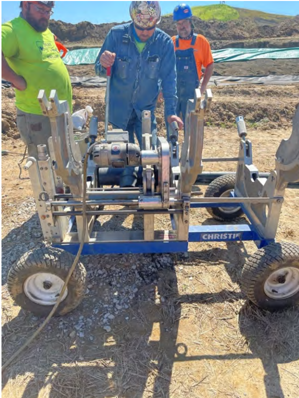
Photo 1: Christie fusion welding machine to replace the McElroy for welding the 4-inch hdpe underdrain pipe at the T section.
