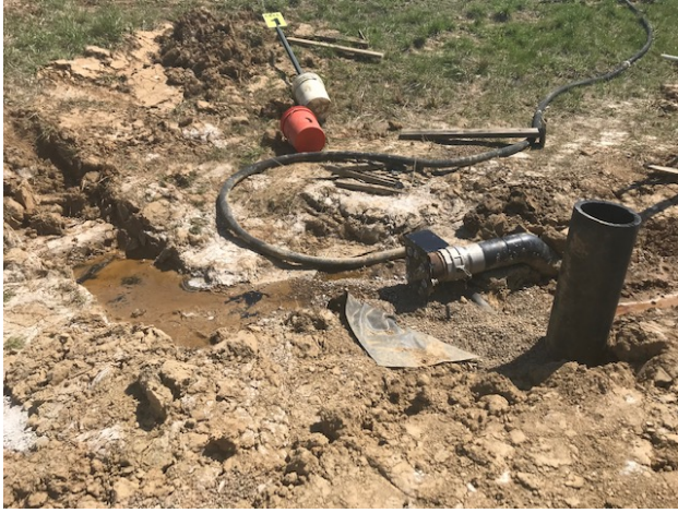
Photograph 8: View of the French drain being built to collect the leachate seepage and direct into the riser pipe. Notice the piece of PVC geomembrane under the French drain stone.
