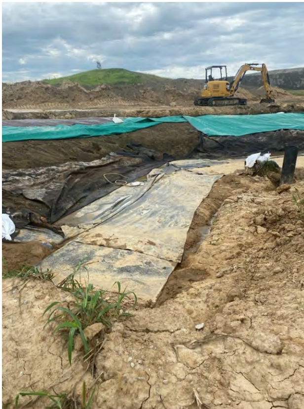
Photo 1: Exposed floor liner and rain flap prior to removal of existing geomembrane.
