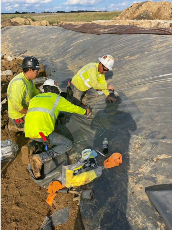
Photo 1: toward the south end CCS continues to replace the thermal welds at the toe of the berm with an adhesive repair.
