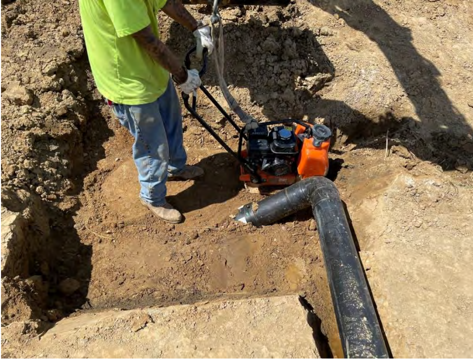
Photo 1: The electrofusion coupling is still visible in this photo. Enerfab has filled in the pipe excavation, and is using a vibrating plate to compact the soil back in place around the pipe.
