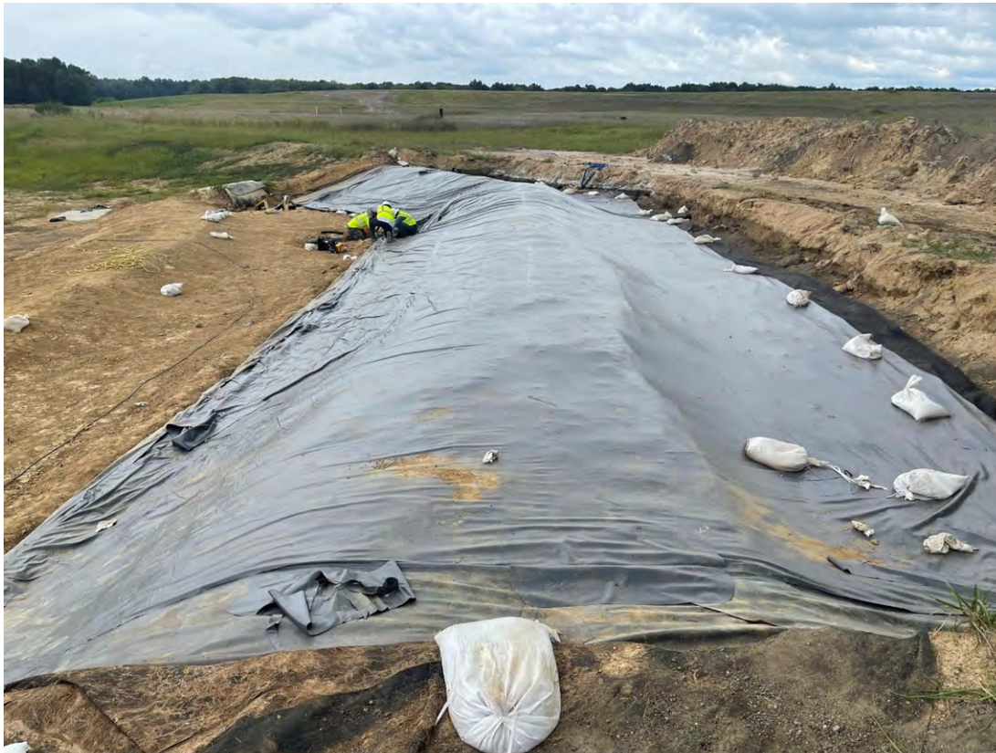
Photo 1: Looking north CCS deployed the PVC liner over the geotextile and bottom ash berm.
