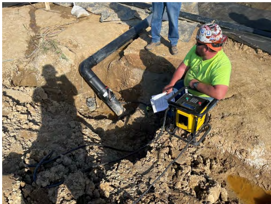
Photo 2: Enerfab is using the thermal coupling equipment to weld the underdrain to the existing leachate line.
