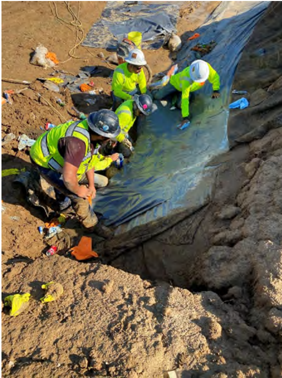
Photo 1: Placing new chemical patch over repaired area on south end of berm.
