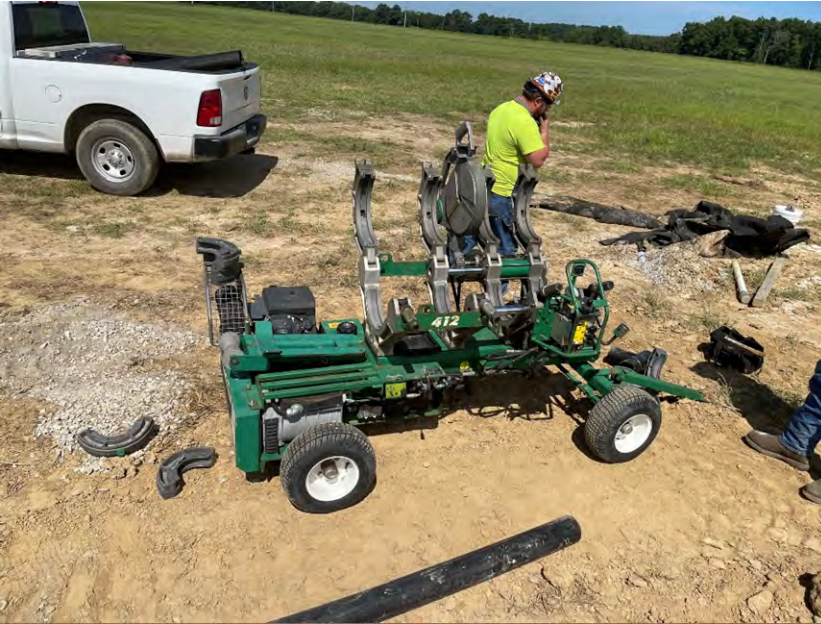
Photo 1: Butt fusion welding machine for 4-inch HDPE underdrain pipe. Machine is a McElroy Pitbull 212/618 HF
