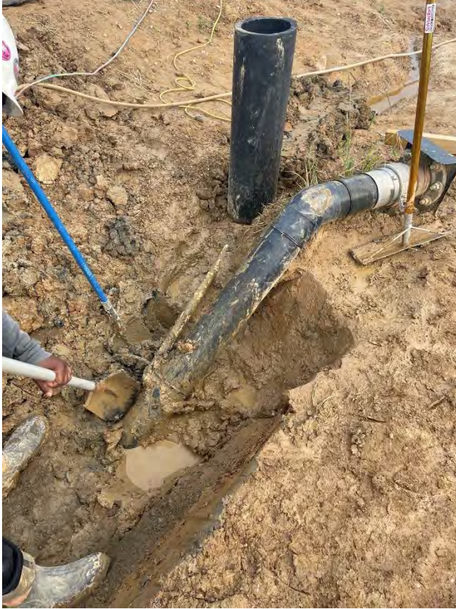
Photo 1: The large-diameter vertical pipe shown was placed temporarily to collect leachate within the construction area.
