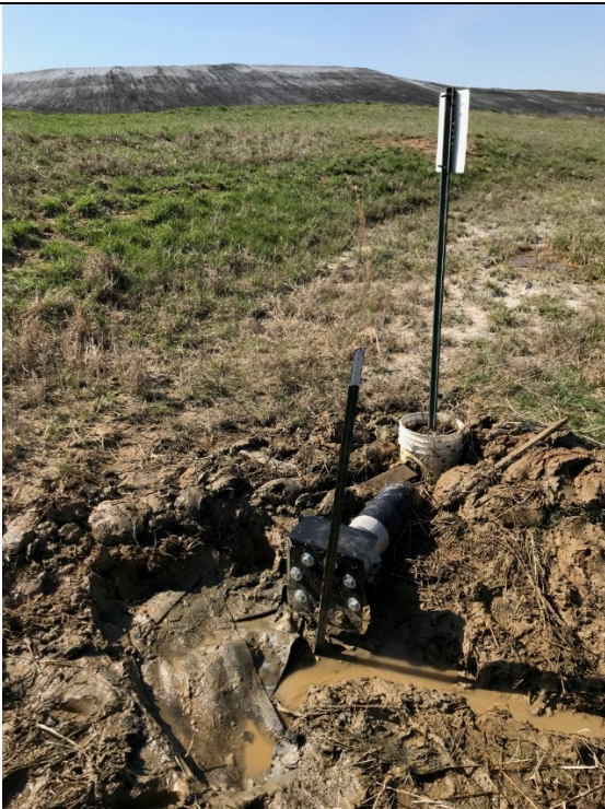
Photograph 2: Another view of the leachate seepage shortly after initial discovery in the area around Quick Connect #12, with the active Phase 1 area in the background.
