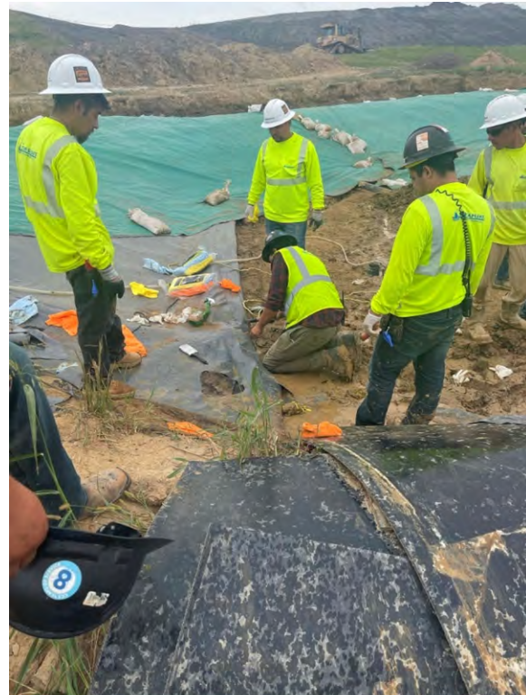
Photo 2: CCS working at the north end of the liner weld between existing and new PVC. The leachate in this area prevented a patch from being made today.
