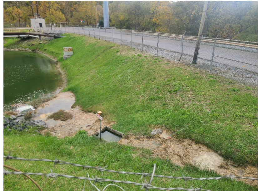
Photo #8 – seepage leading towards weir #5
