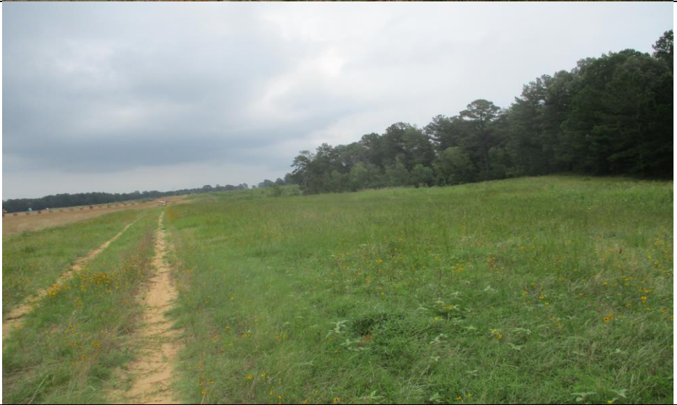
Photograph No. 16 Typical view of the south dike of the upstream slope.
