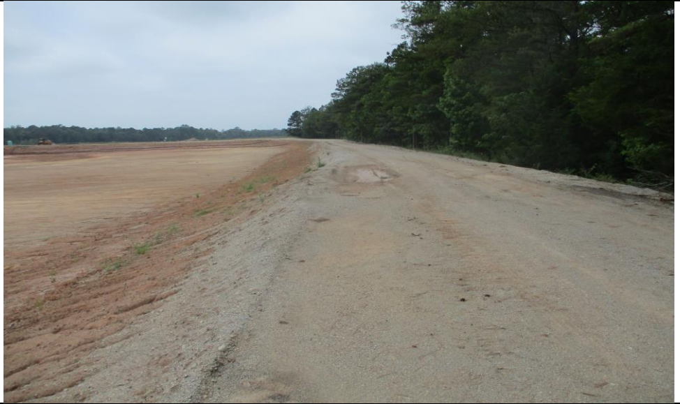
Photograph No. 9 Minor rutting at the crest.
