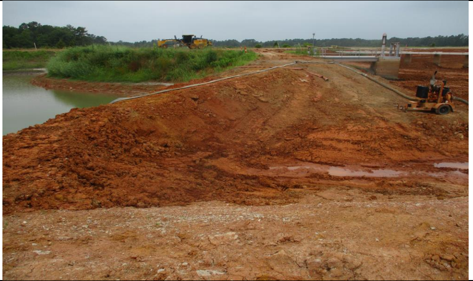
Photograph No. 3 Portion of the dike excavated due to pond closure activities.
