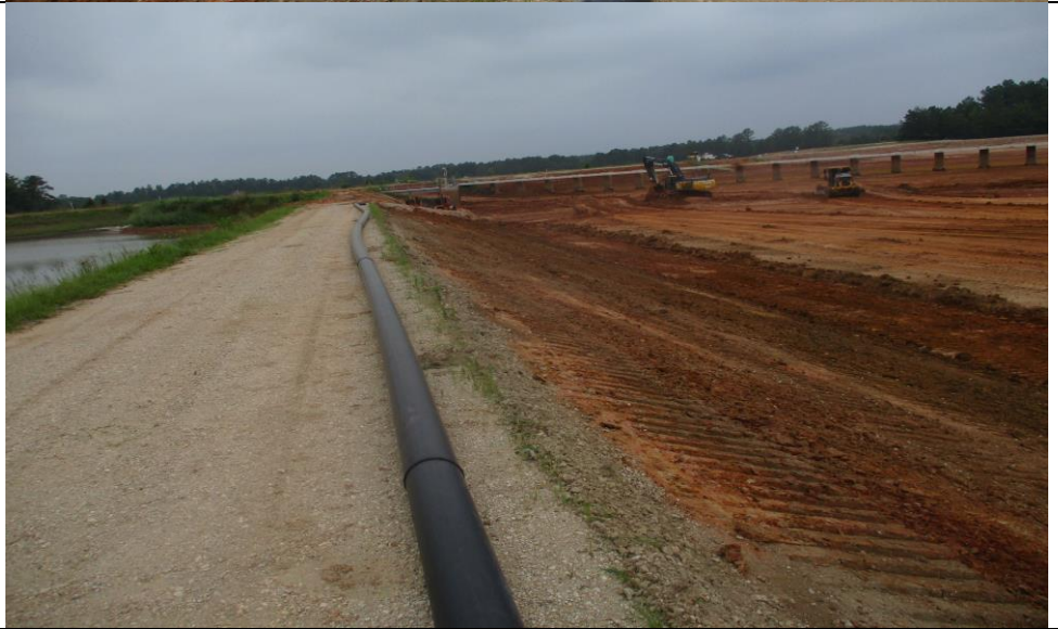
Photograph No. 2 View of the south dike crest and upstream slope (looking west).
