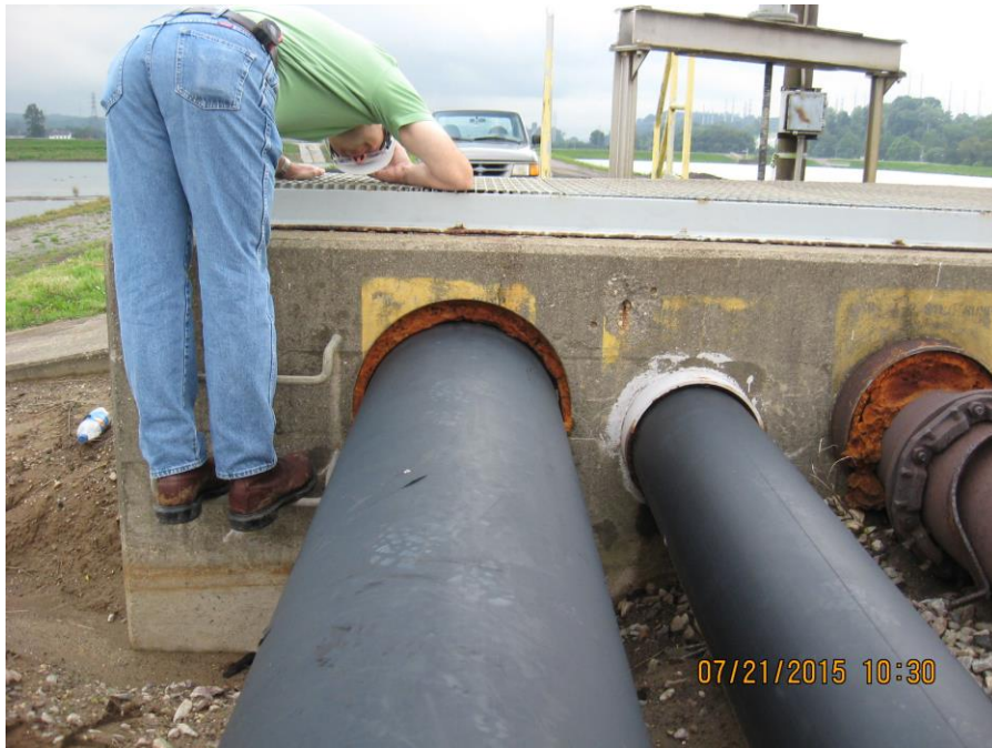
Photo 8: Bottom Ash Ponds: bottom ash inlet pipes and inlet structure.
