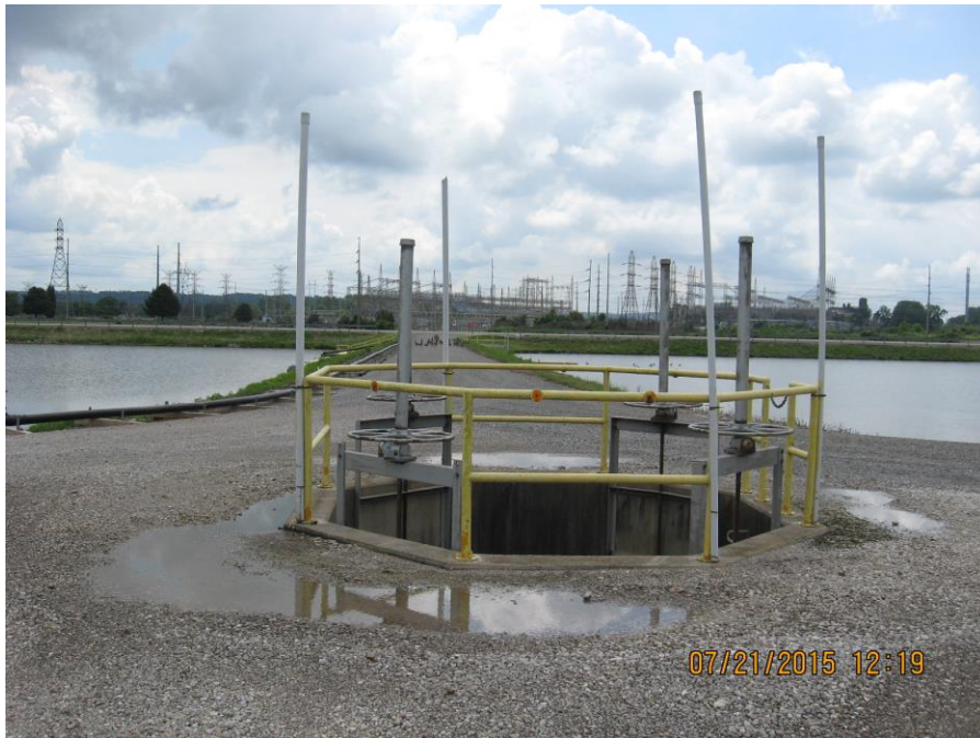
Photo 58: Waste Water Ponds: valve outlet structure.
