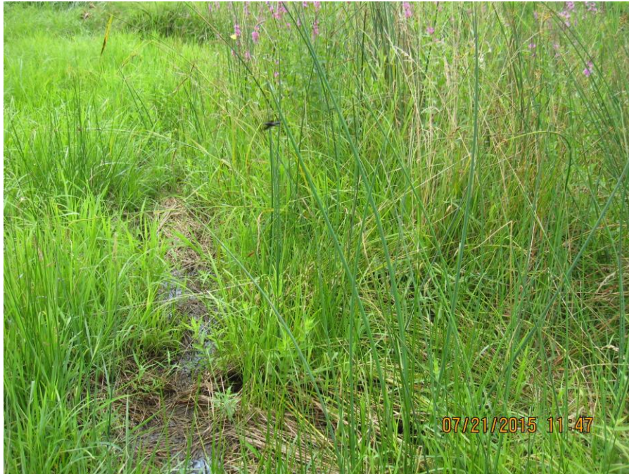
Photo 47: East Wastewater Pond, east dike: water along exterior toe.
