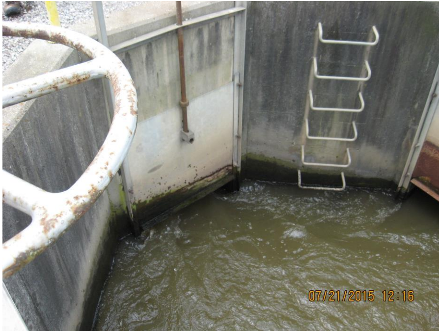
Photo 59: Waste Water Ponds: valve outlet structure.
