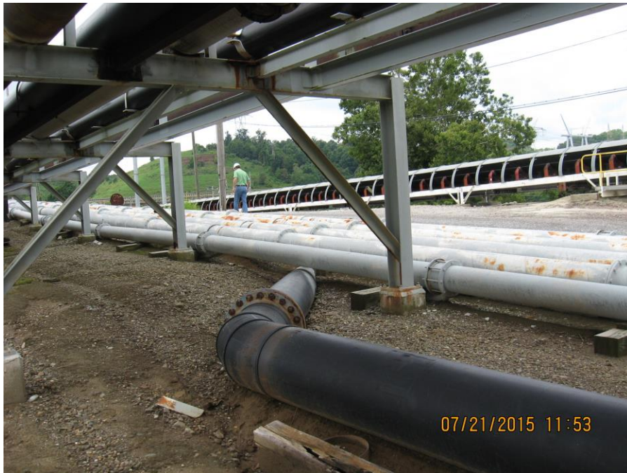
Photo 51: East Bottom Ash Pond, north dike: bottom ash inlet pipes.
