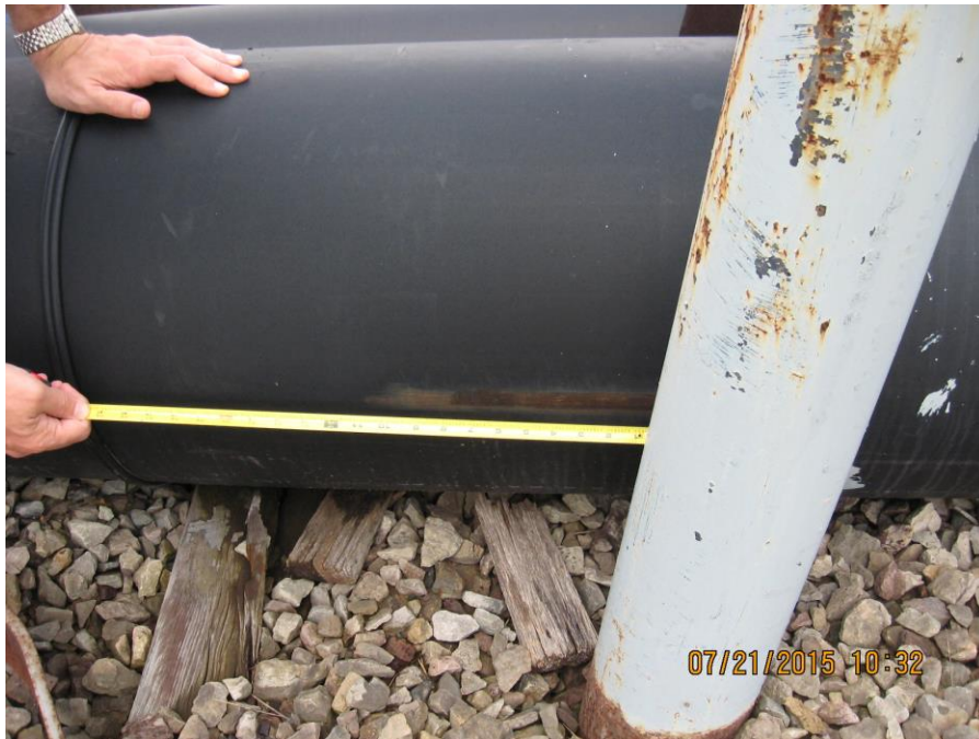
Photo 9: Bottom Ash Ponds: evidence of movement along bottom ash inlet pipes due to thermal expansion.
