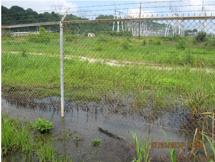
Photo 17: Bottom Ash Ponds, north dike: water near the exterior toe.
