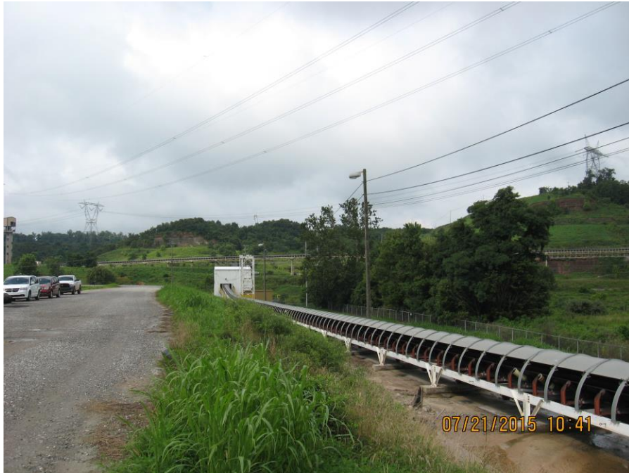
Photo 13: Bottom Ash Ponds, north dike: gypsum conveyor.
