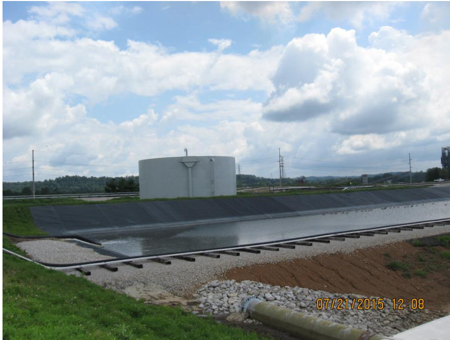
Photo 57: Leachate Surge Pond.
