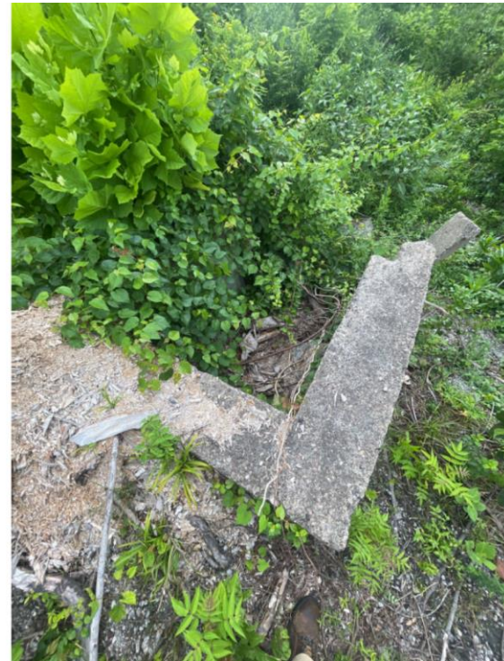
Media 34: Remnants of old concrete outlet structure used when the ash pond was active
