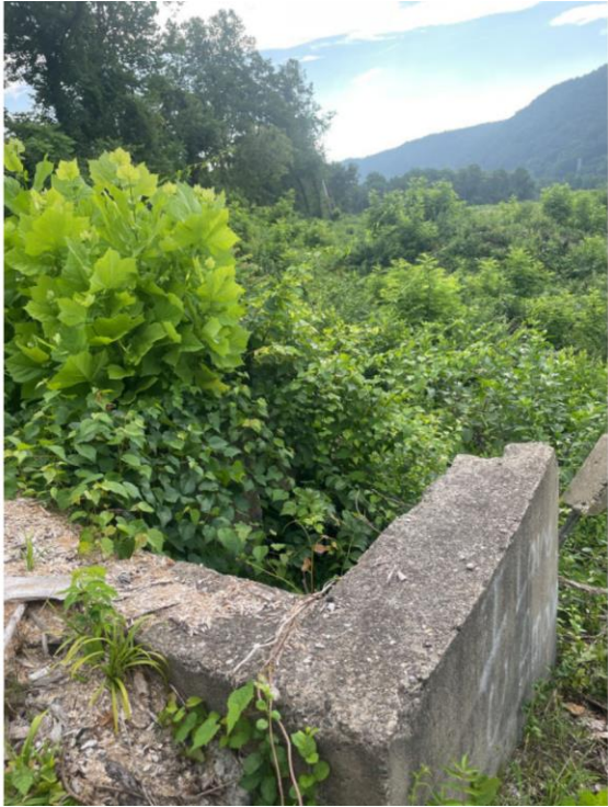
Media 35: Remnants of an old concrete outlet structure used when the ash pond was active
