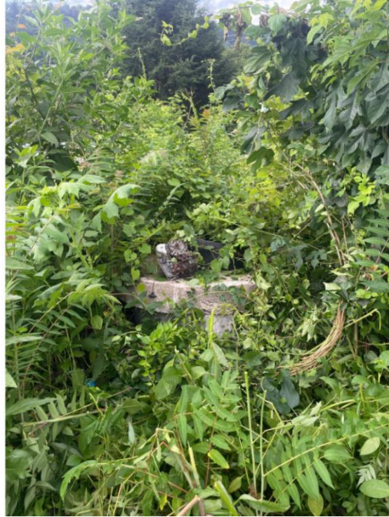
Media 42: Top of concrete stormwater manhole. Access point for stormwater drainage pipes that traverse the ash pond
