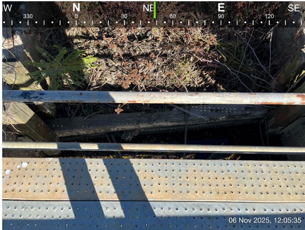
Photograph 9. View of stop log weir separating northern and southern ash pond basins.
