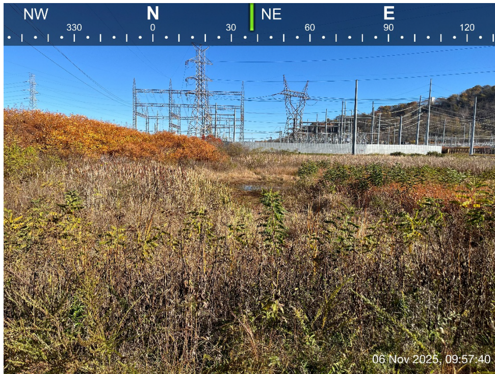
Photograph 5. View of Kammer 345 kV Station.
