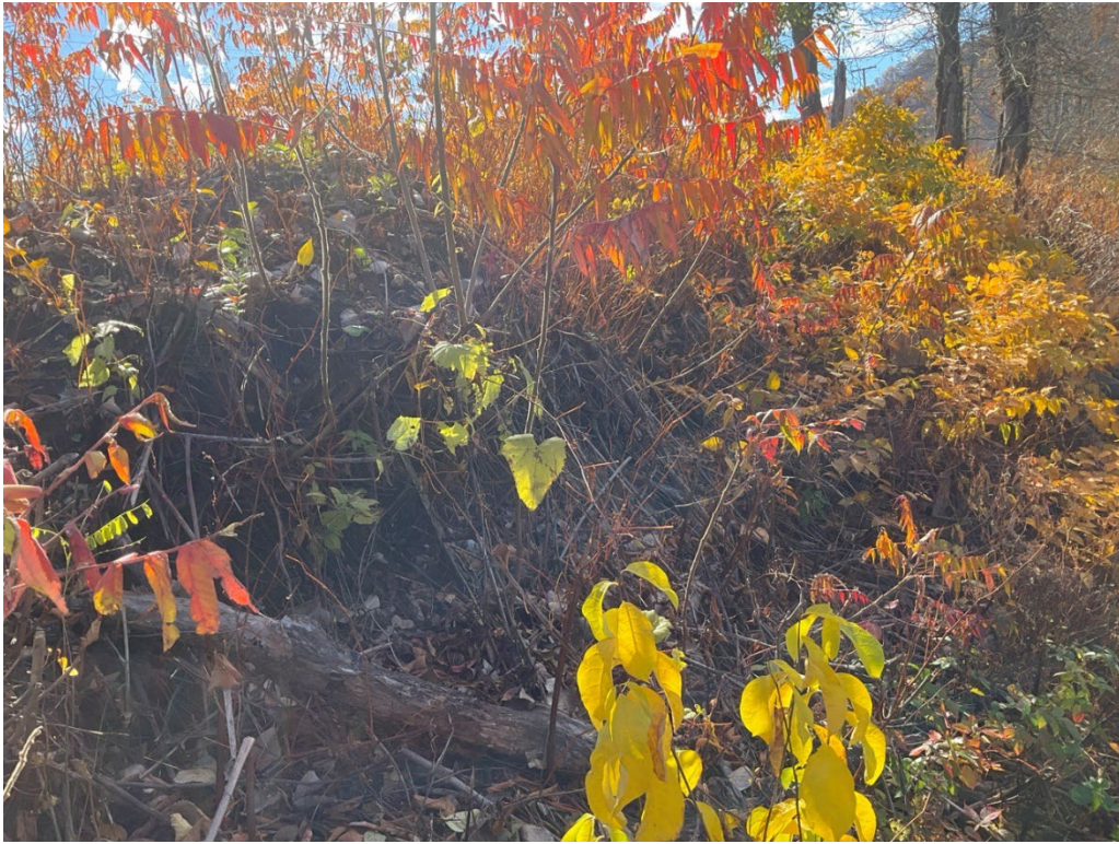
Photograph 7: View of the exterior dike slope looking south. Note surface erosion.
