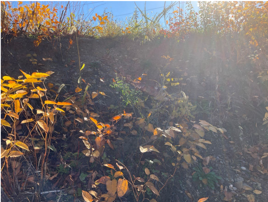
Photograph 4: View of the exterior dike slope looking north. Note surface erosion.
