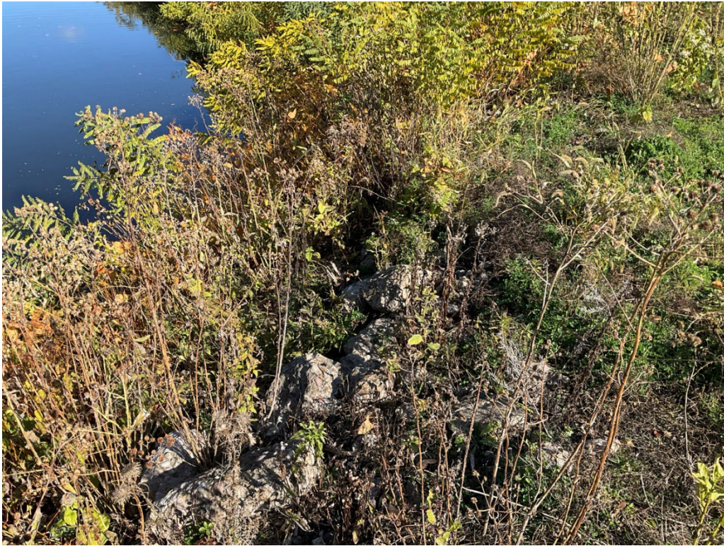
Photograph 11: View of the interior dike slope looking north. Note concrete debris.
