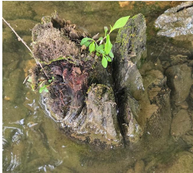
Figure 3-4: Pile 9 of Subzone B1 with large vertical separation between remaining segments (left and right sides)
