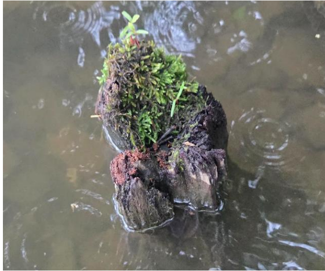
Figure 3-1: Typical pile conditions with only decayed heartwood remaining above water.
