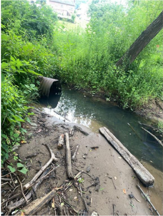
Media 29: Corrugated metal storm drain outlet
